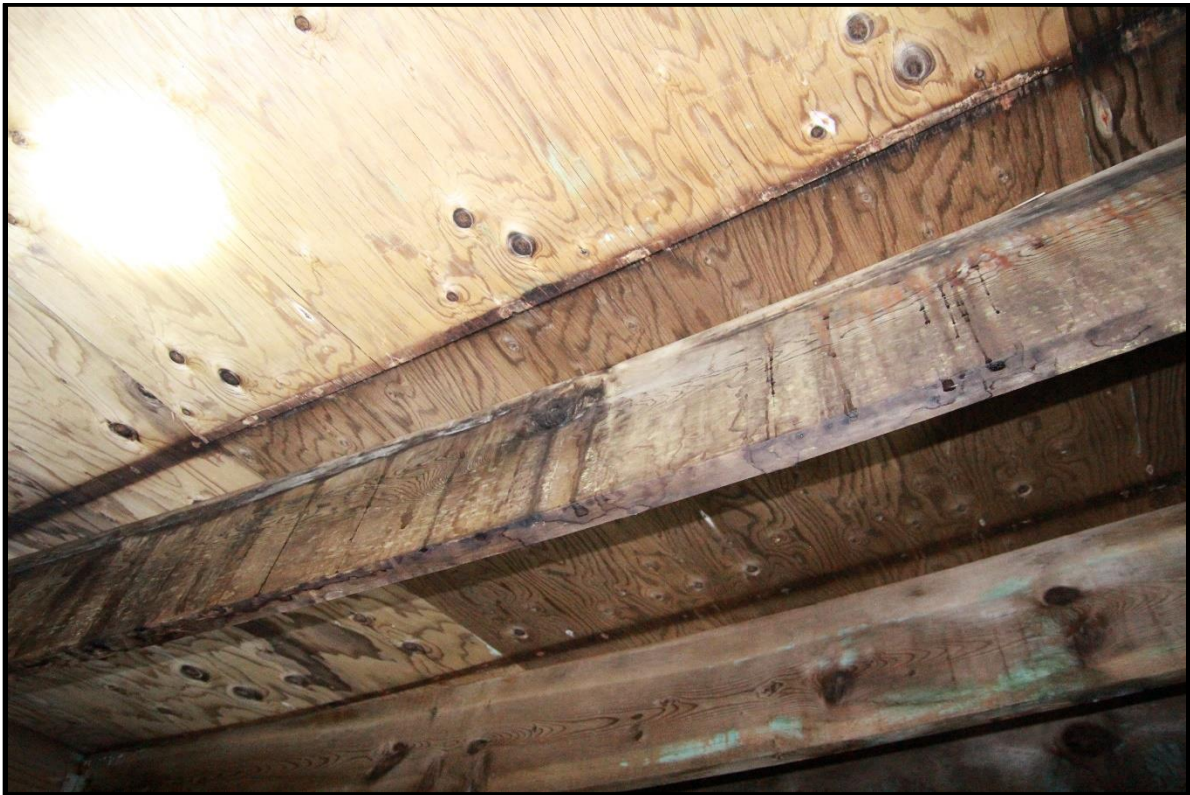
Unsupported Sheathing Due to Joist Deflection
