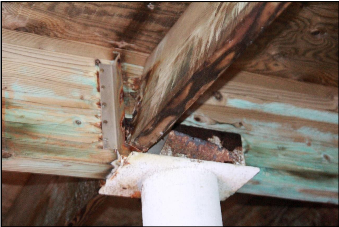
Failing Joist And Hanger
