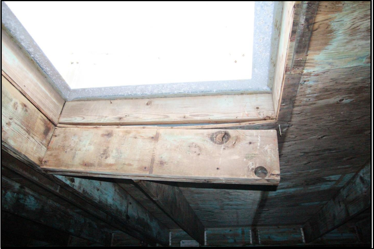
Roof Joist Missing Due To Failed Hangers
