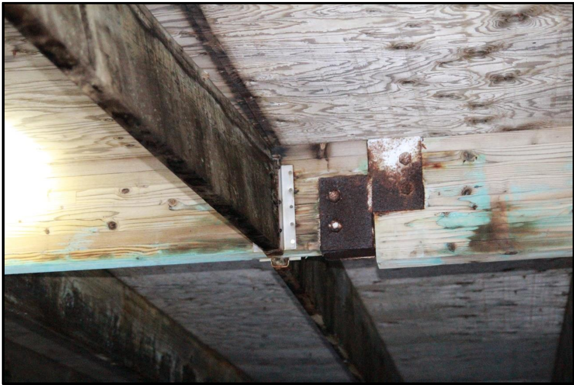
Failing Splices and Joist
