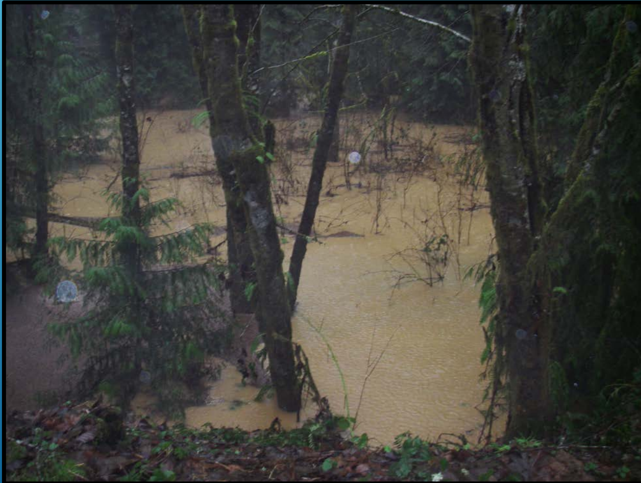
Impounded water at access road culvert
