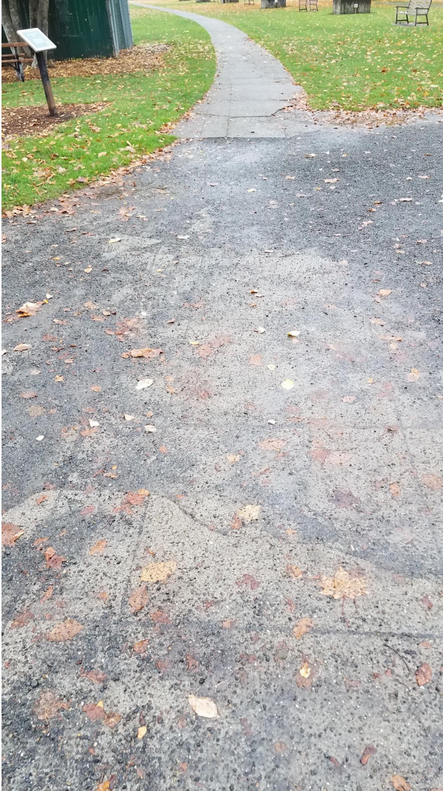
Photo # 12: Existing sidewalk not proposed to be replaced (located in the main part, damaged, and covered with gravel)
