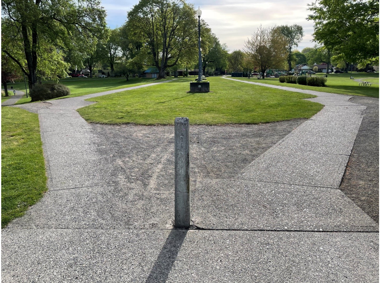
Photo # 4: Near the pedestrian bridge, project stops outside of the panel with the bollard
