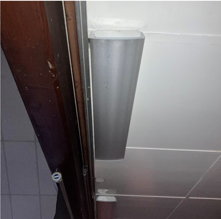
Stage lights. Bulbs to be replaced with LED.
