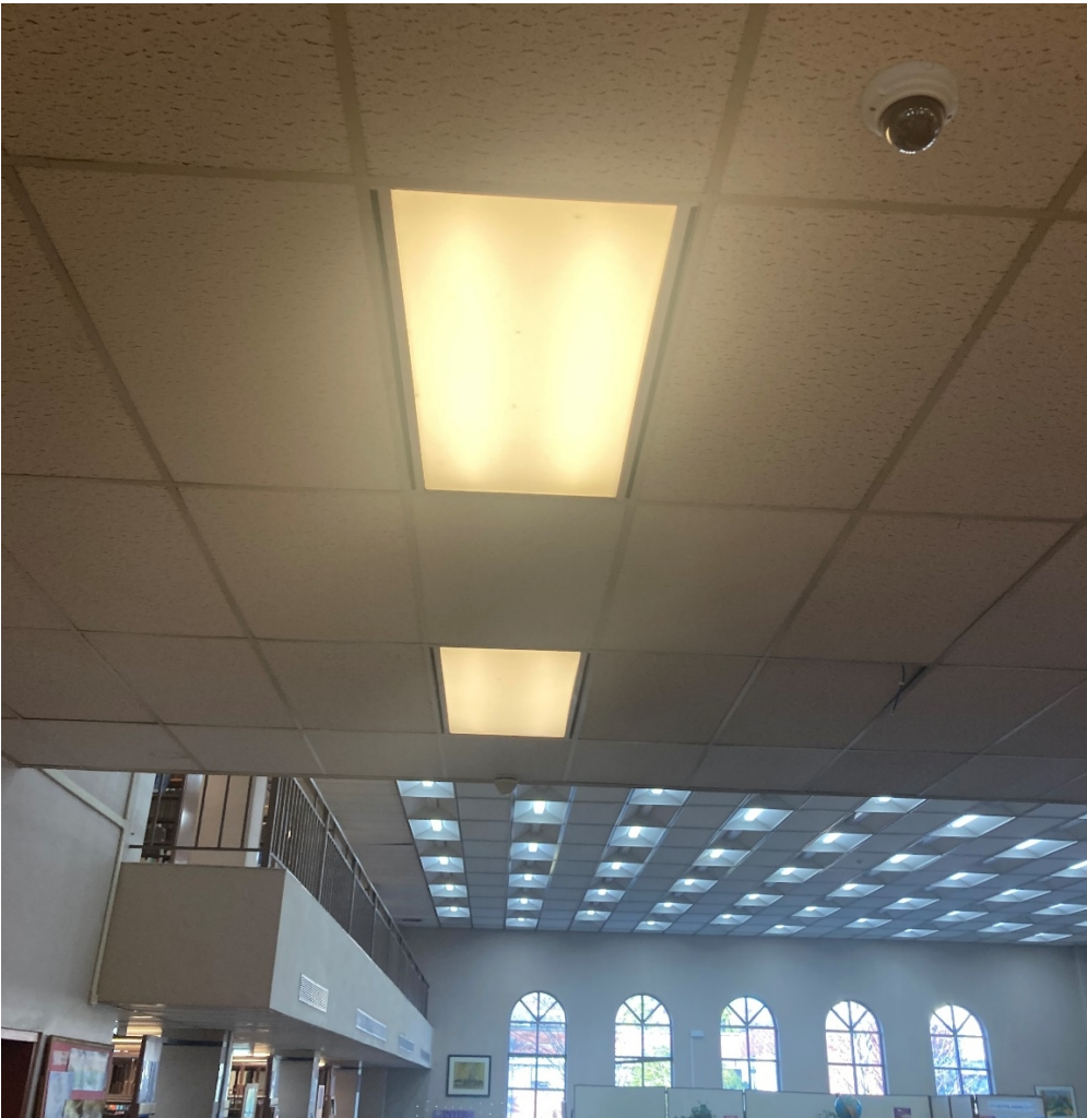
Fluorescent fixtures through out to be converted to LED bulbs.
