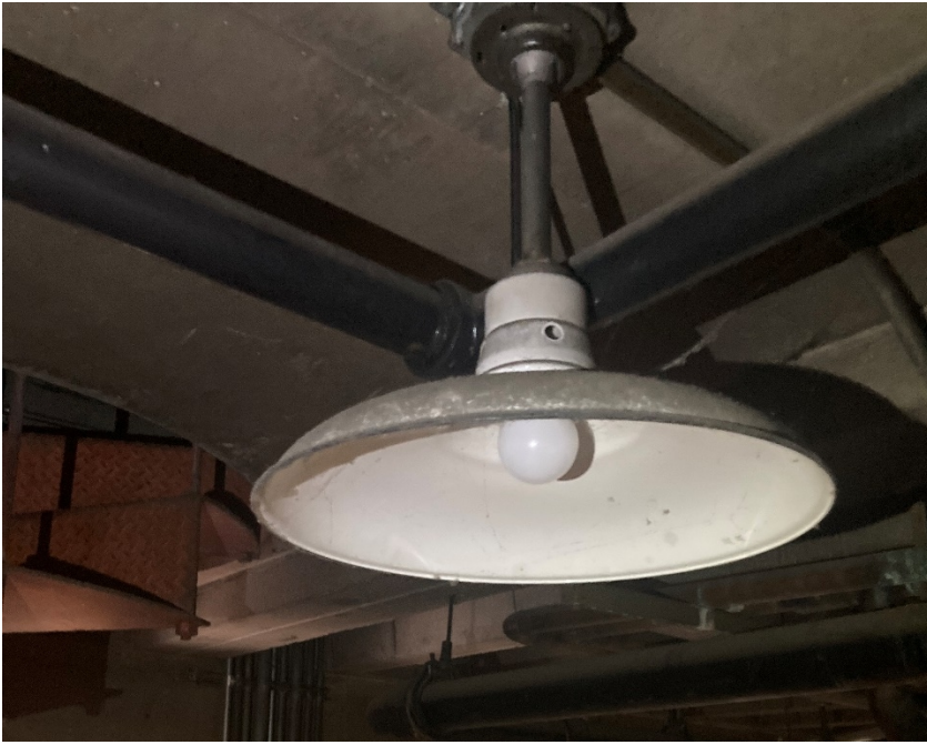
Mechanical Room. Bulbs to be replaced with LED.
