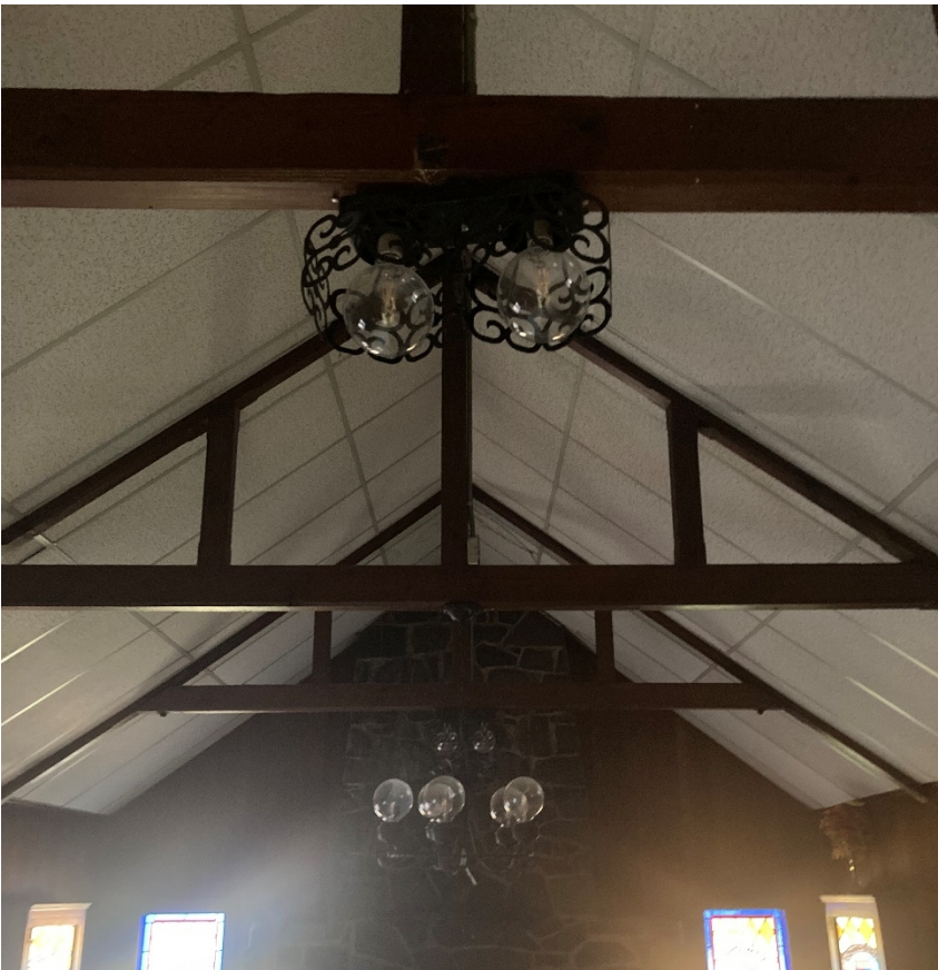
Existing Main room fixtures. Previously, converted to LED.
