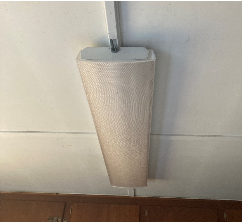
Hallway lights. Bulbs to be replaced with LED.
