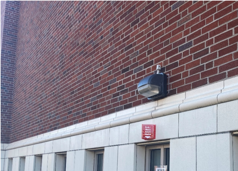
Exterior fixtures to be replaced with LED fixtures.
