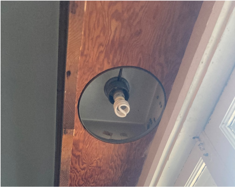
Kitchen fixture, bulb to be replaced with LED.
