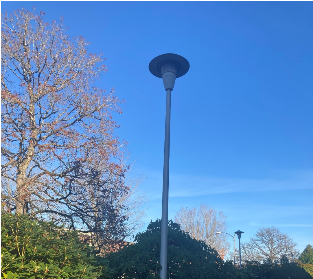
Parking lot lighting heads to be replaced with LED fixtures.
