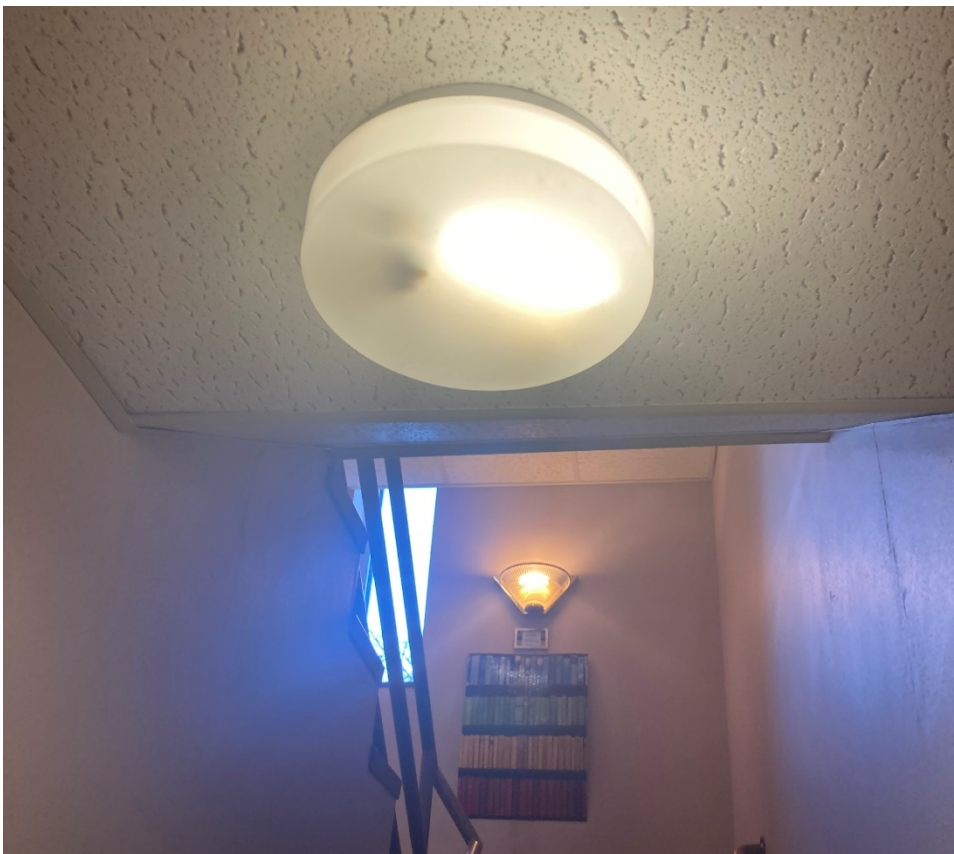
Stairwell lighting. Round fixtures to be replaced with LED. Sconce to get LED bulbs.
