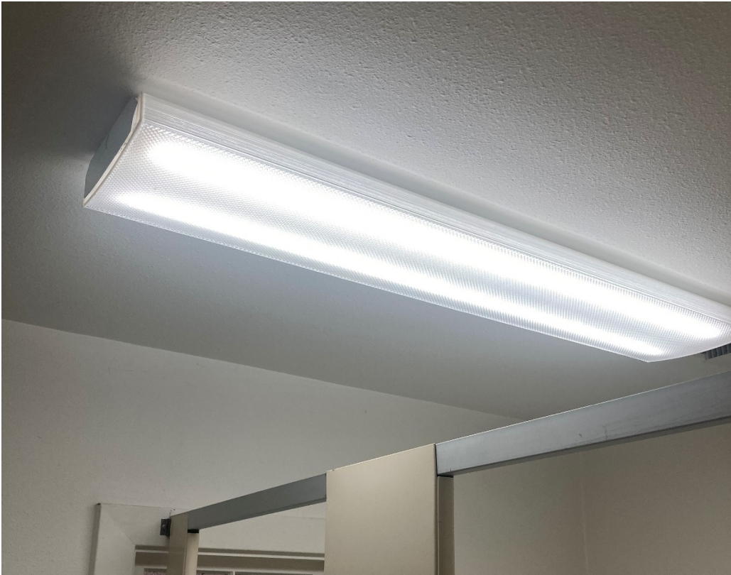
Bathroom lights. Bulbs to replaced with LED.
