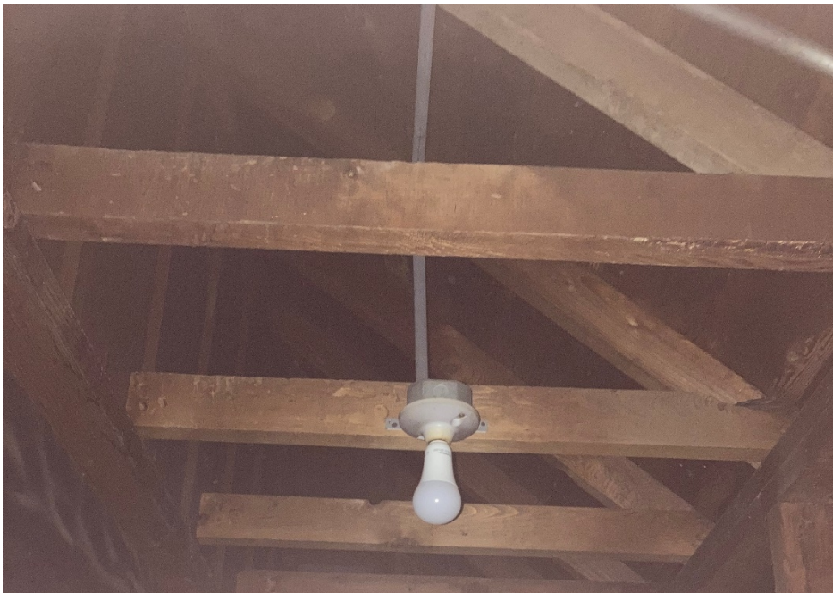
Basement Fixtures. The bulbs that are not already LED will be replaced with LED.
