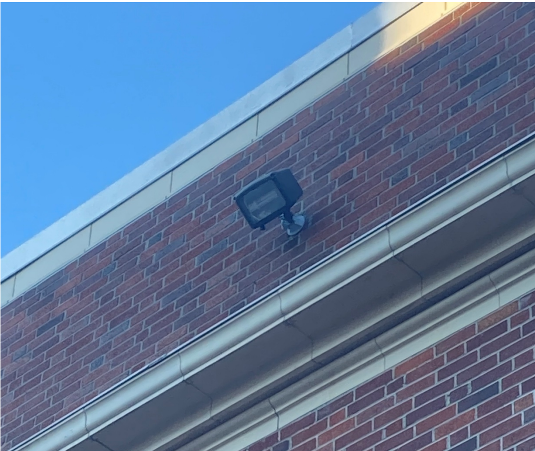
Exterior Fixtures to be replaced with LED.
