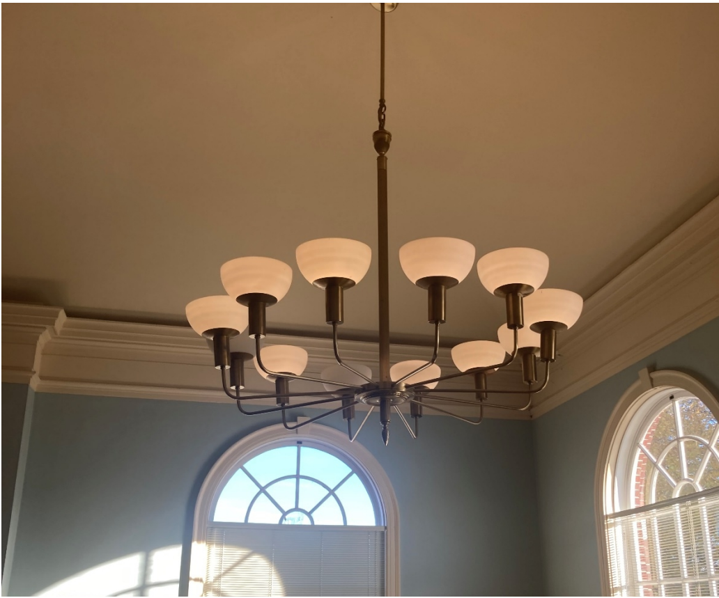
Chandeliers to be converted to LED bulbs. Potentially rewired and sockets updated.
