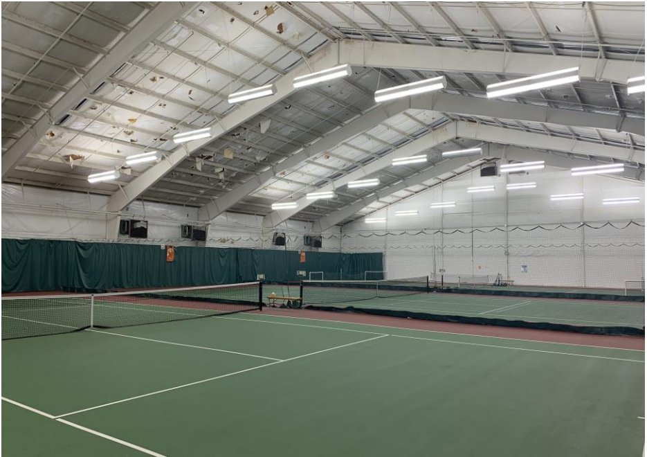
Damaged ceiling over the MVFC tennis courts
