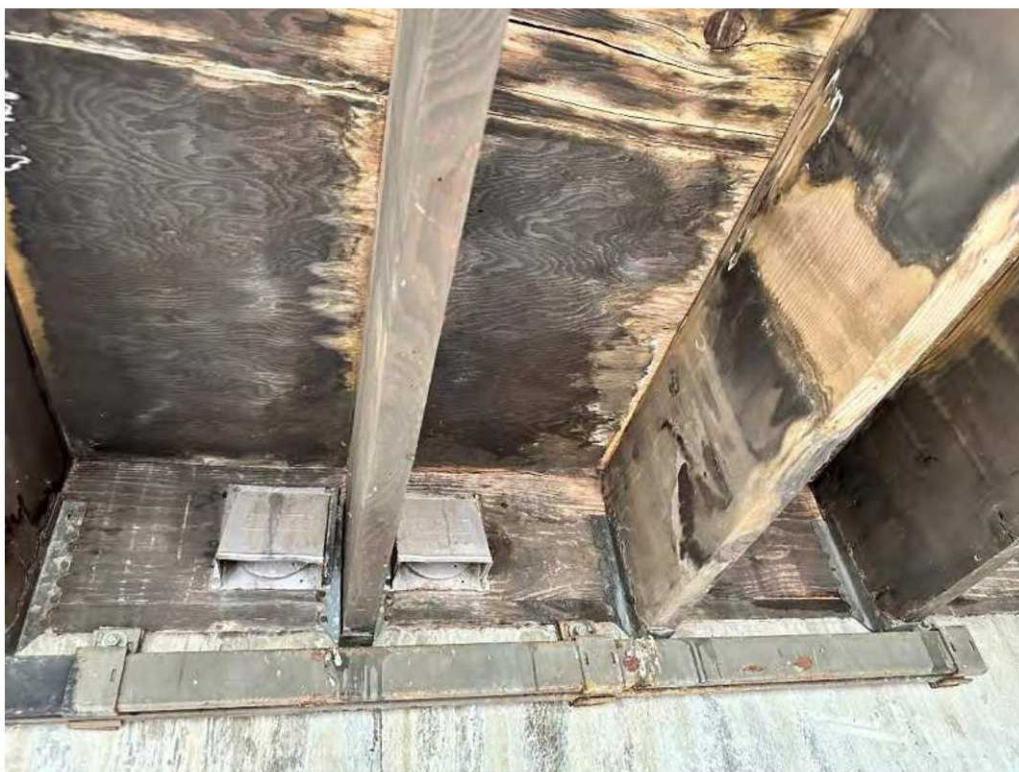
Water damage under concrete patio
