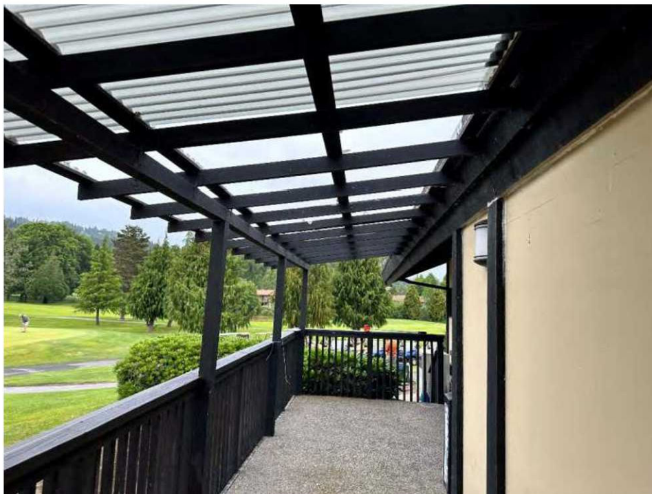
Missing panels on the overhang above the back patio
