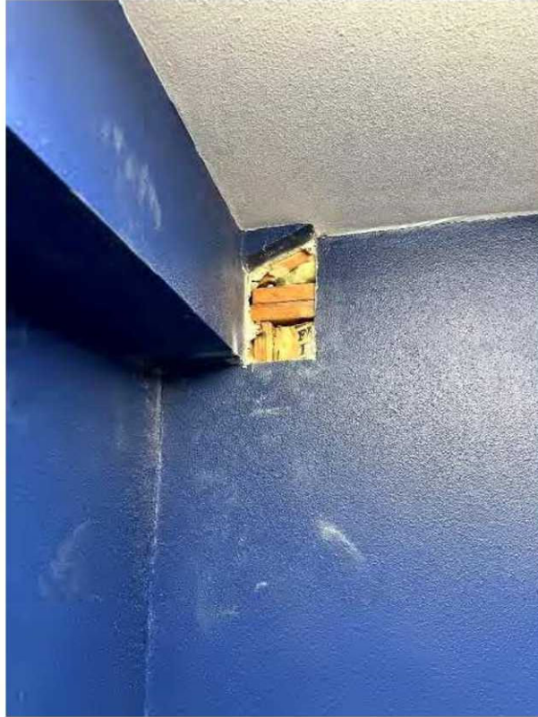
Women's bathroom sheetrock and insulation damage
