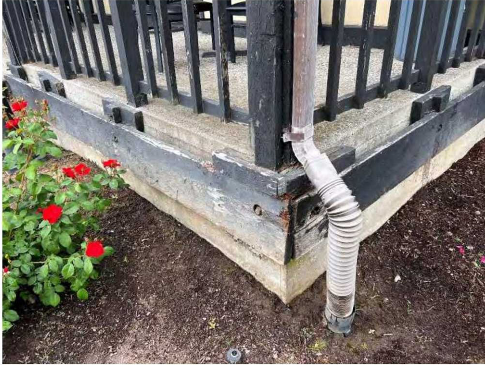
Decorative exterior siding around back patio showing signs of rot
