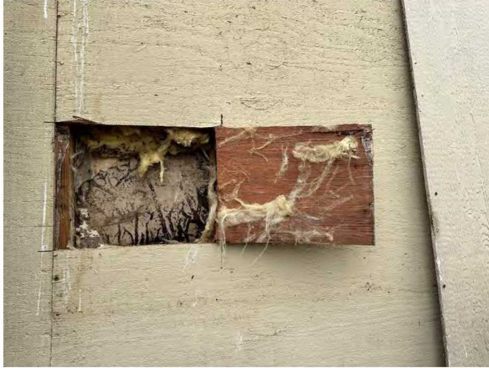
Inside of bathroom wall from exterior showing signs of mold growth and bug infestation
