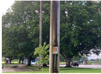
Roy Morse Light Poles - Electric Boxes & Holes
