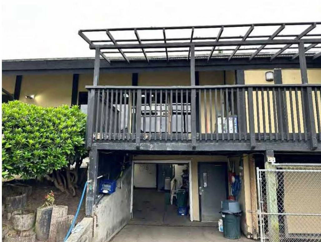
Sagging beams holding up concrete patio
