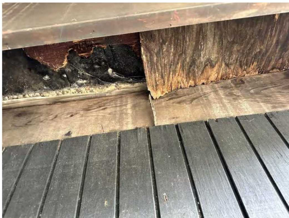
Deck rot under concrete patio
