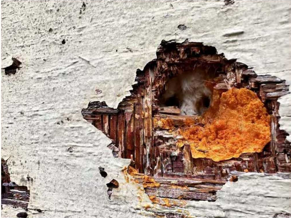
Close up of hole on exterior bathroom siding
