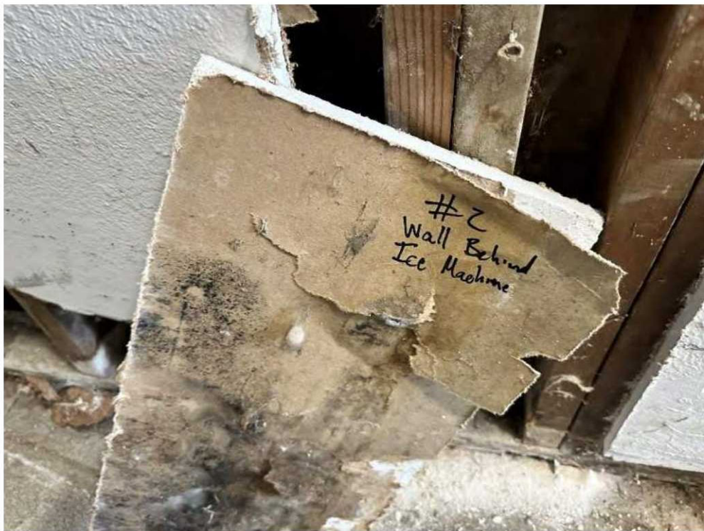
Mold growth on sheetrock behind basement ice chests
