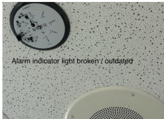
Station Alerting System 4
