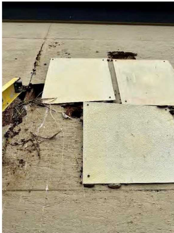
Large area of exterior siding rot damage behind bathroom walls
