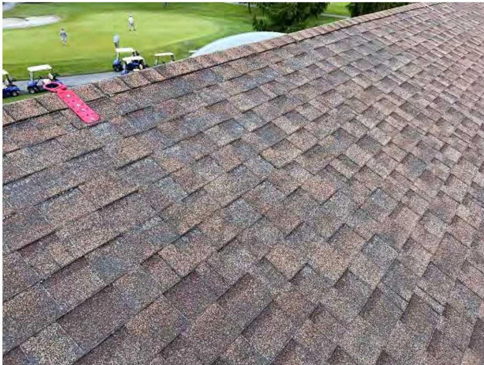
Degradation and missing granules on the shingles
