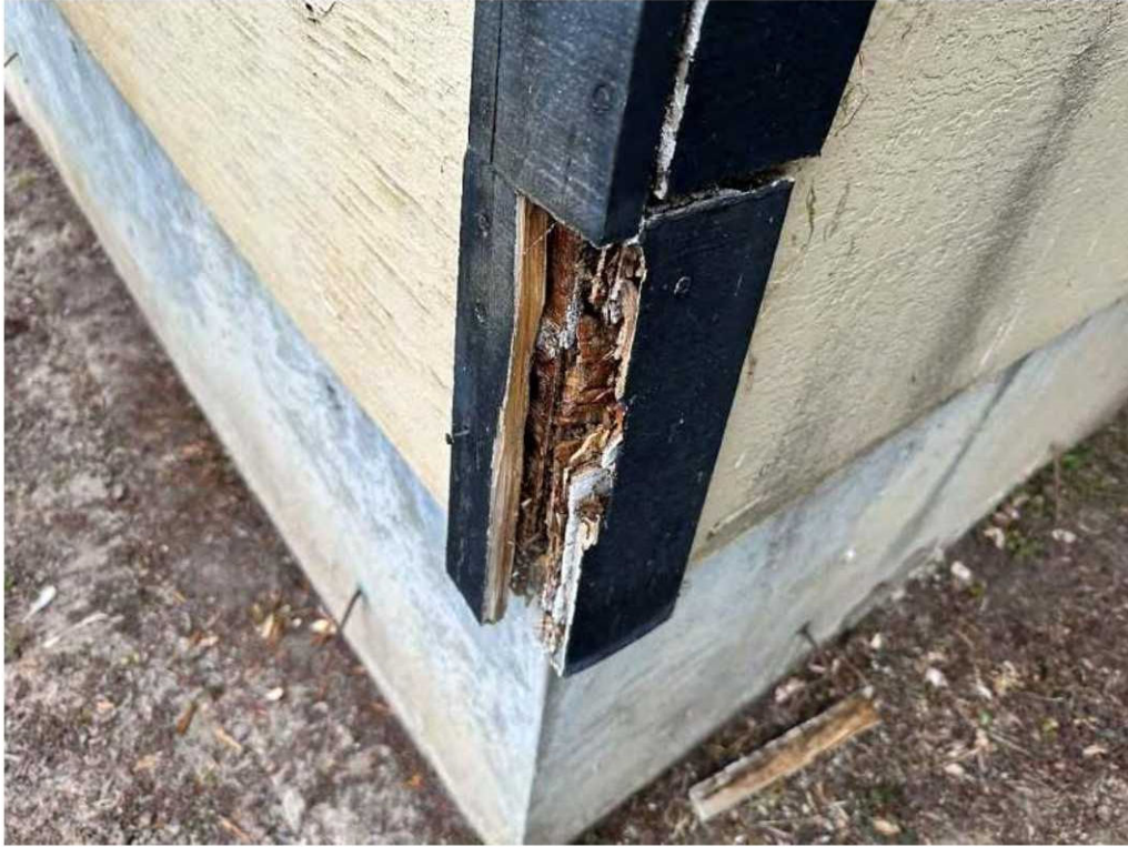
Trim on exterior bathroom siding has also begun to rot away
