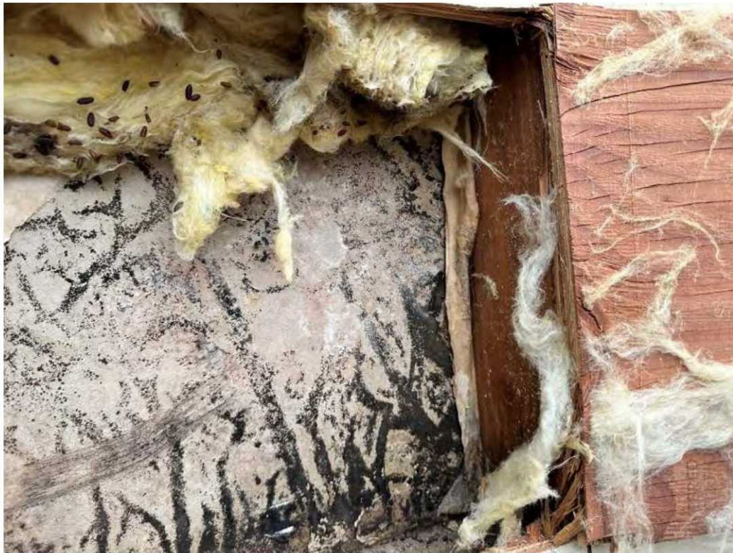
Inside of bathroom wall from exterior showing signs of mold growth and bug infestation
