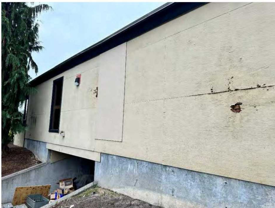
Exterior bathroom siding has degraded away in many places causing holes allowing for moisture to enter
