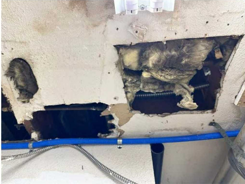
Downstairs storeroom ceiling showing water damaged sheetrock
