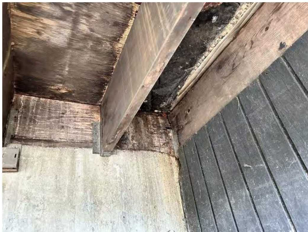
Deck rot under concrete patio
