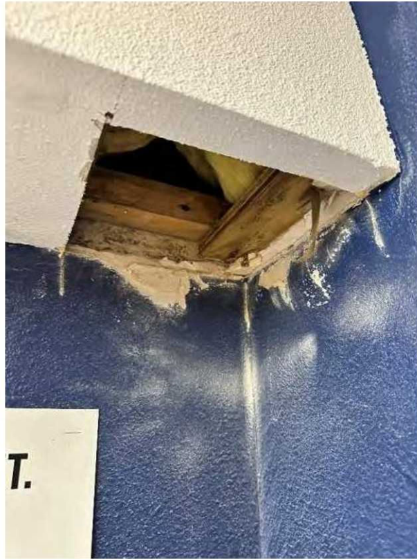
Men's bathroom sheetrock and insulation damage
