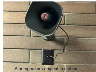
Station Alerting System 3
