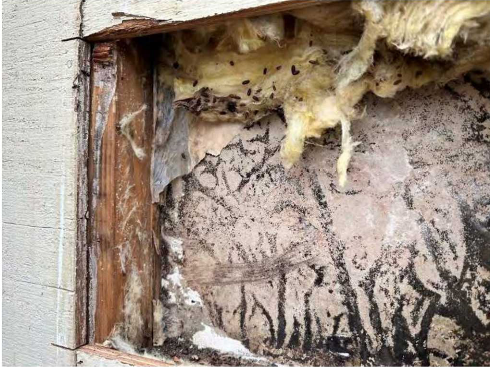
Exterior wall outside men's bathroom showing mold growth
