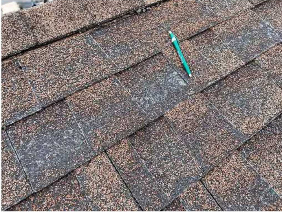
Degradation and missing granules on the shingles
