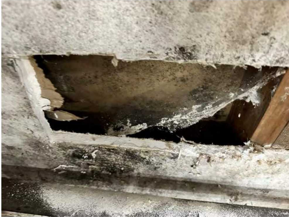
Water damaged sheetrock behind basement ice chests
