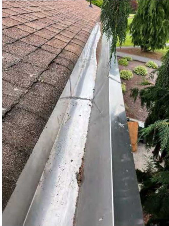
Inside of gutter could be sealed to prevent future leaks
