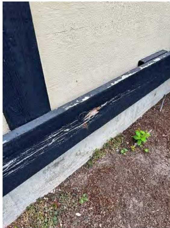
Decorative exterior siding beginning to rot away behind sales wall
