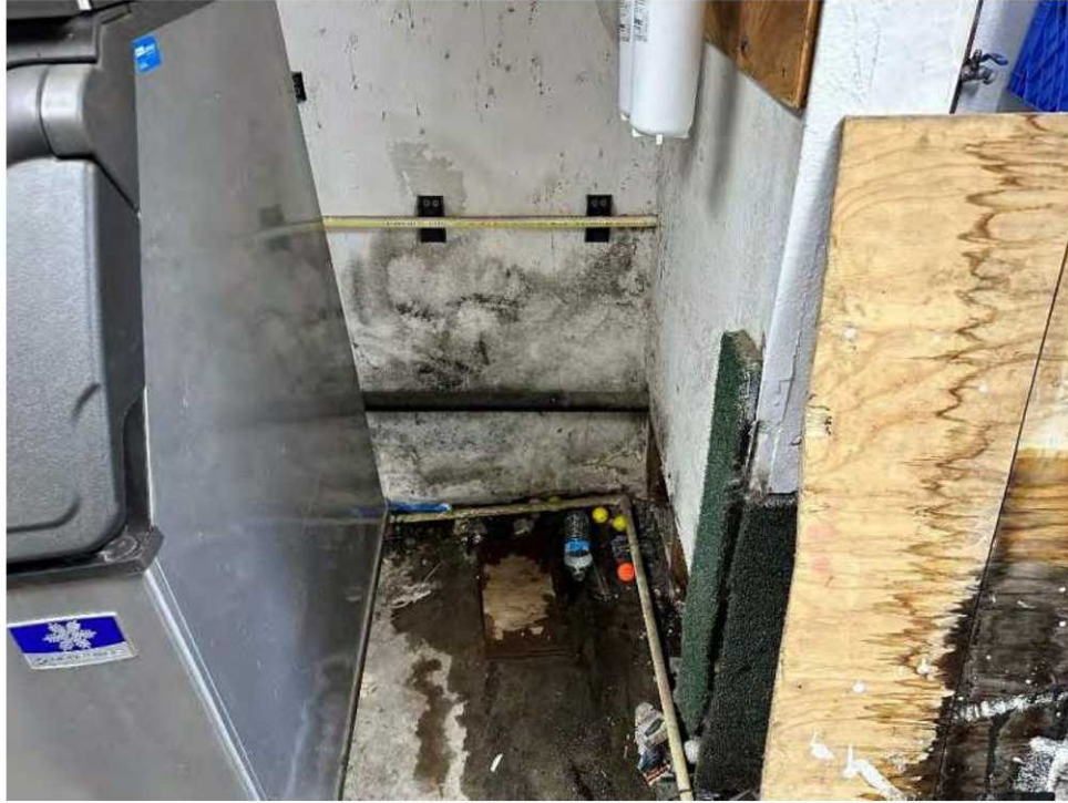
Wet sheetrock behind ice chests in basement
