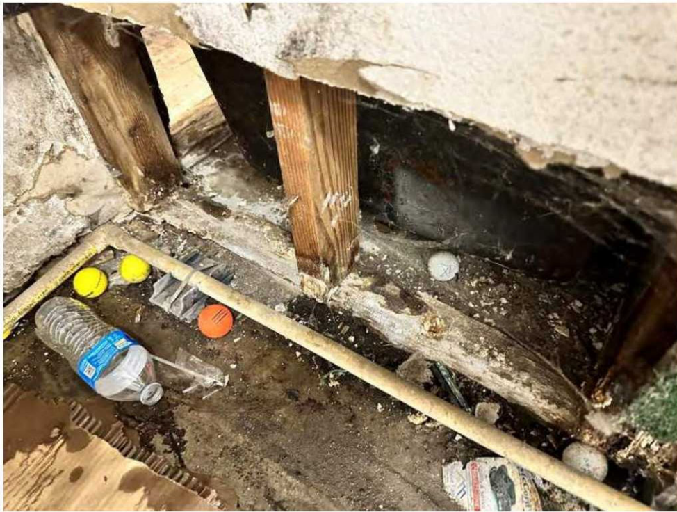
Water damaged framing behind ice chests in basement
