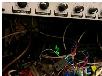
Station Alerting System 1
